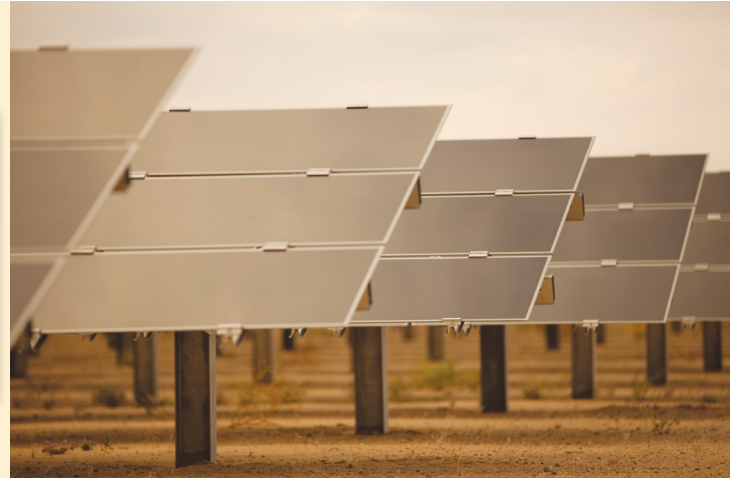
Solar photovoltaic panels at NRG's Blythe Solar Project
